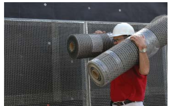
The two rolls carried by this worker contain enough, PermaLath 1000 to cover nearly 1,000 square feet
